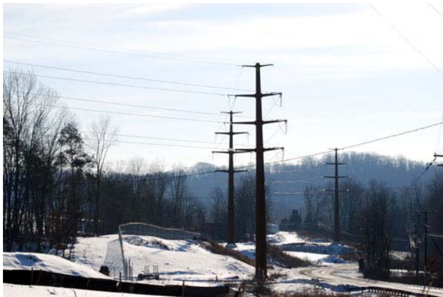
January 2011 High voltage towers along Route 519
