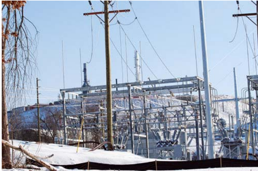
New Allegheny Power substation will provide electricity for expanded processing activities in 2011 and beyond
