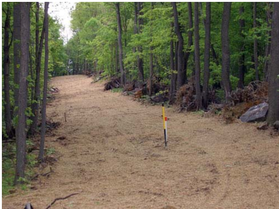
One of the many gas pipelines running into the MarkWest plant
